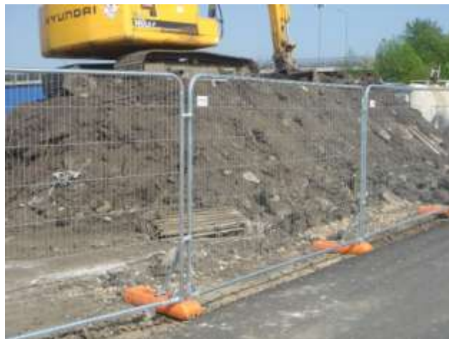
Open mesh type fencing
