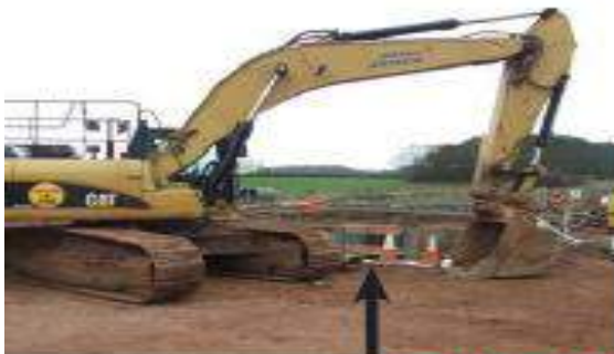
Ground Worker struck here when the bucket moved suddenly towards the cab
