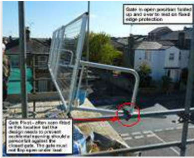
Photo 3: Gate in open position folded up and over to rest on fixed edge protection
