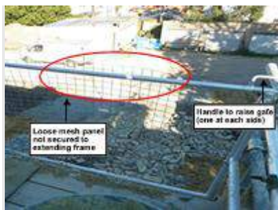
Photo 2: Loose mesh panel not secured to extending frame
