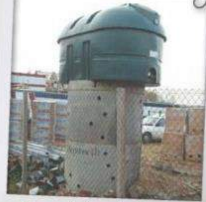
How not to install an oil storage tank!
