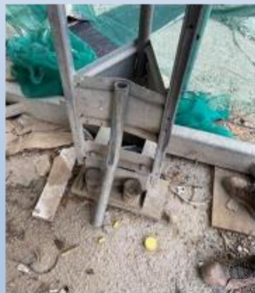
Bad housekeeping by site resulting in damage
